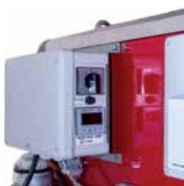
Switch box ISA 65.
